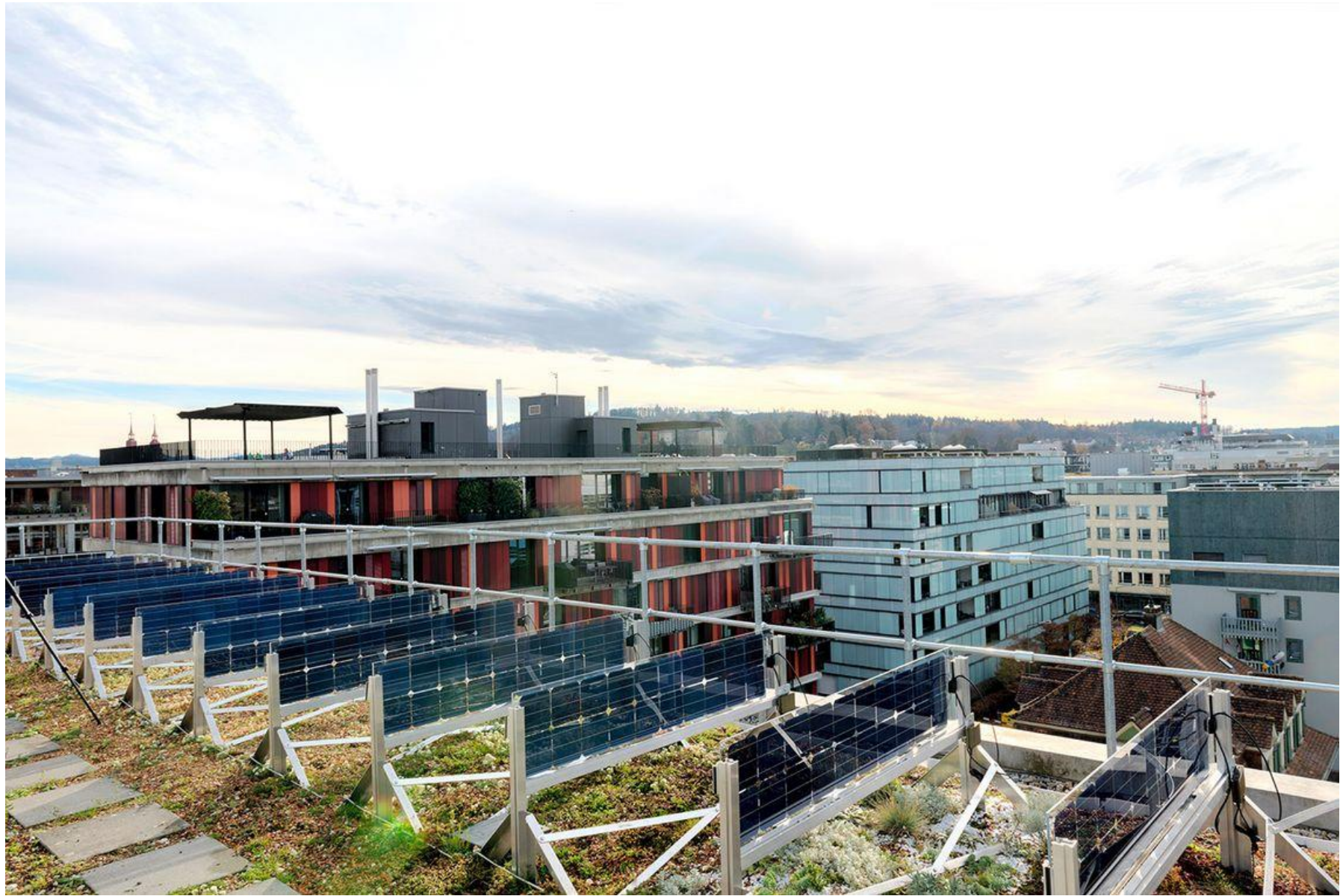
Vertical Bifacial Biosolar Green Roof
