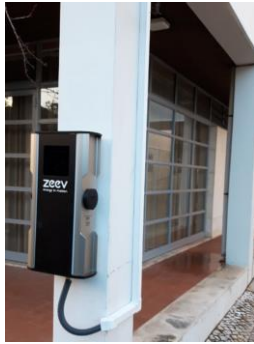
EV Charging station
